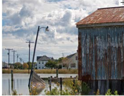
Some of the damage to homes and infrastructure on Hooper's Island from Hurricane Isabel in 2003 has yet to be repaired. (Photo by Erica Goldman.)
