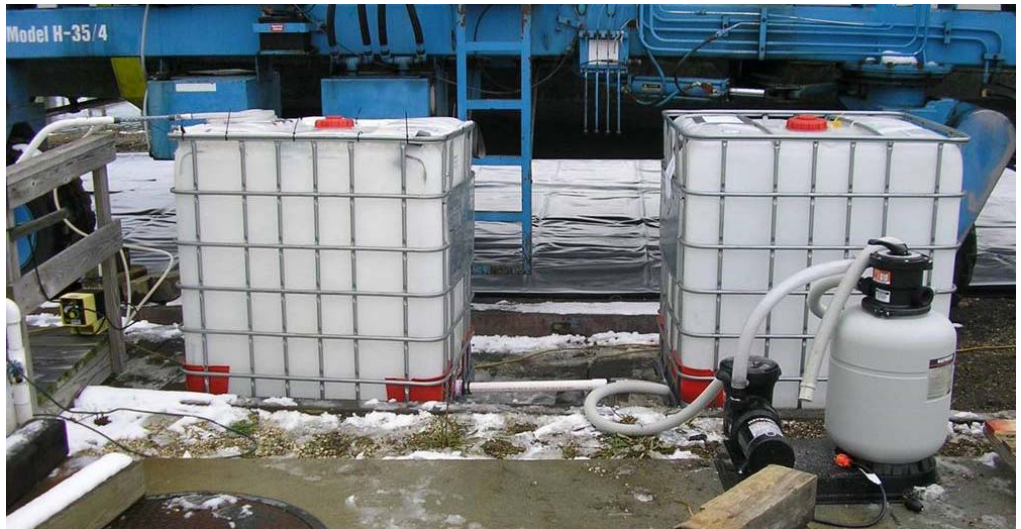
The complete wash wastewater treatment system
