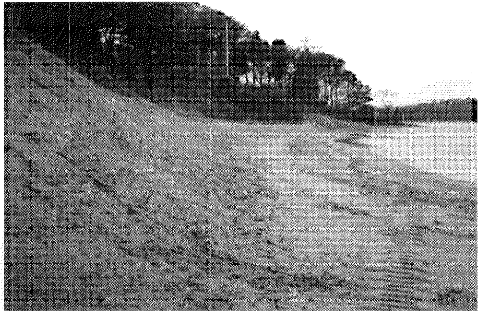
Fig 35. Fiber rolls covered with sediment
